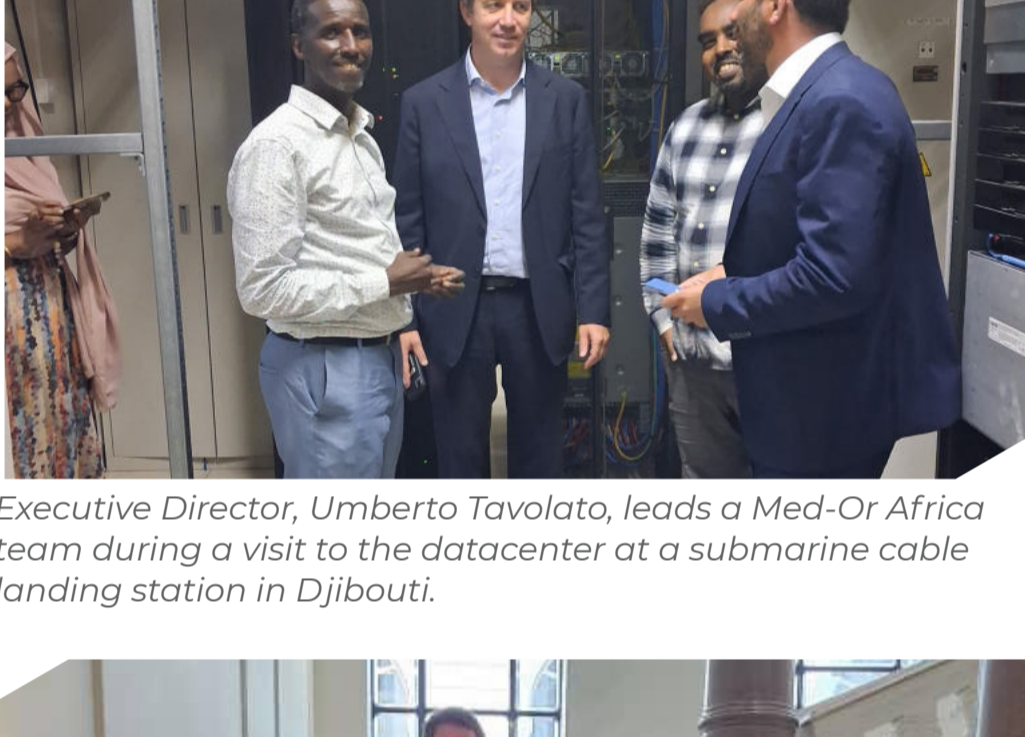
Executive Director, Umberto Tavolato, leads a Med-Or Africa team during a visit to the datacenter at a submarine cable landing station in Djibouti.
